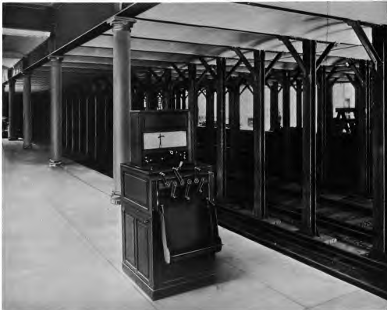
ELECTRO-PNEUMATIC INTERLOCKING MACHINE ON STATION PLATFORM
